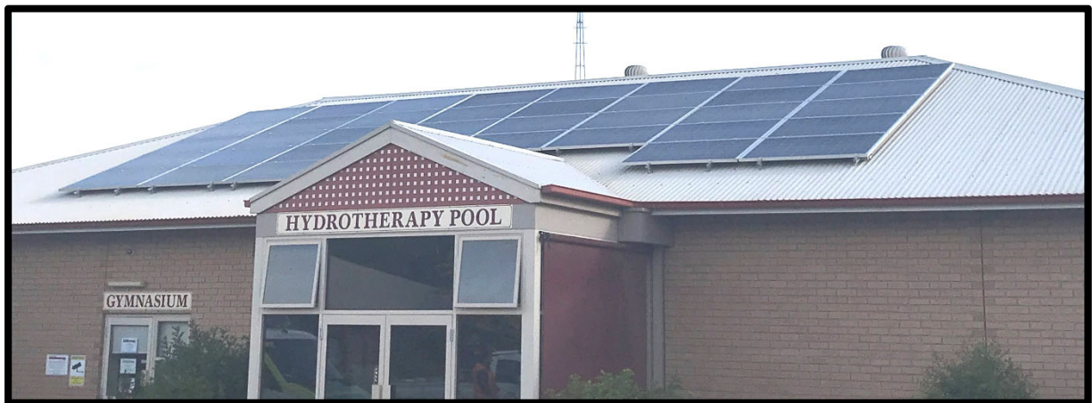
An expansion of the Solar Energy Installation, combined with existing energy efficiency measures has saved significant ongoing expenses at the Regional Hydrotherapy Pool in Jamestown
