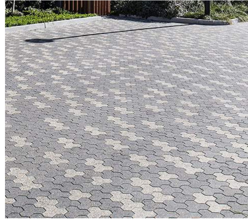
Concrete unit paver (permeable) As required surrounding existing trees within car park verge
